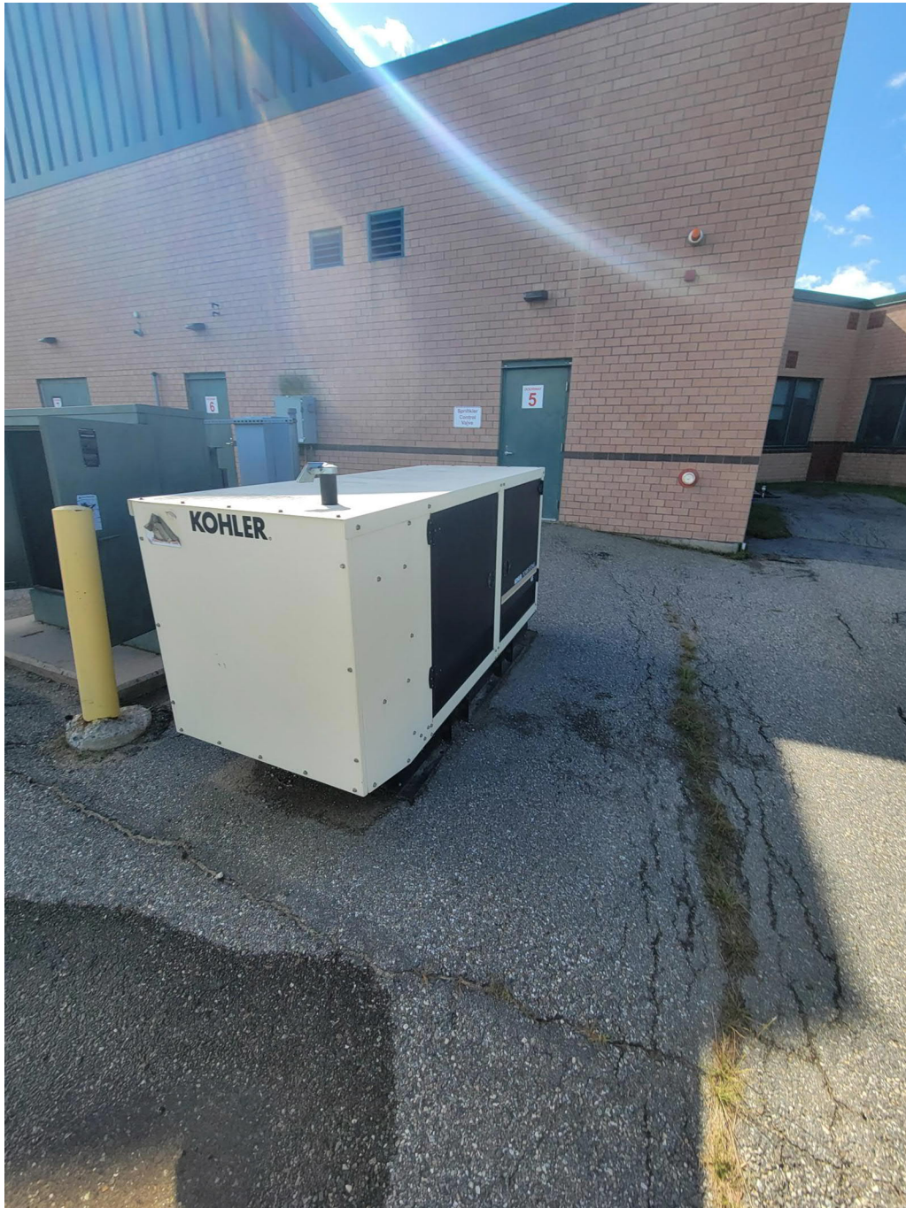
Figure 4 Standby Power Generator
